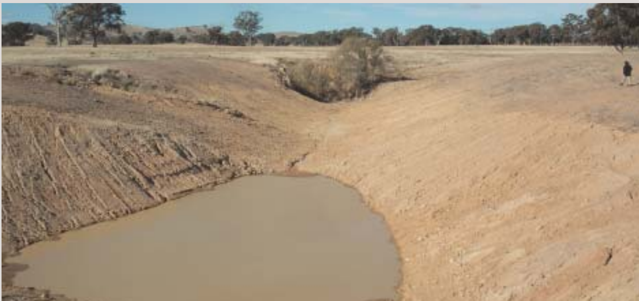
A new dam at Bogolará created in the former deep gully, May 2006. Photo Fleur Flanery.
