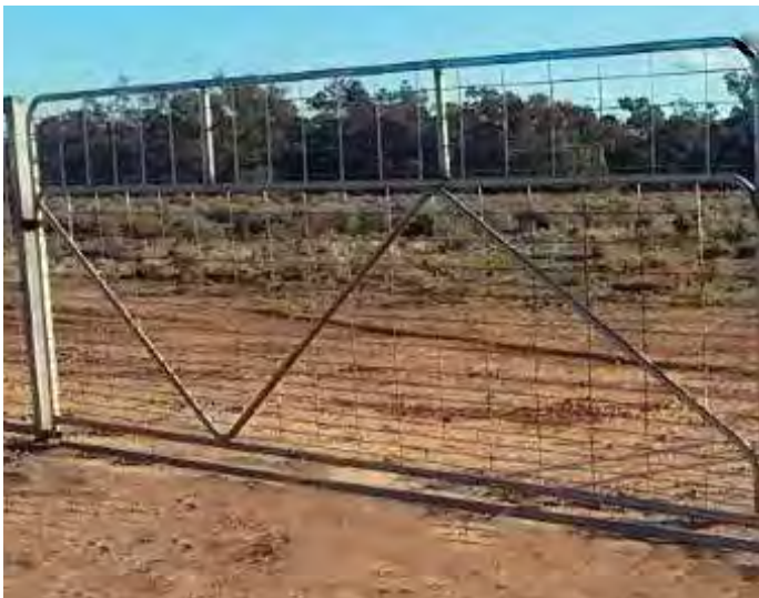
This gate has been designed to minimise the gap between the gate and the posts, and the gate and the ground. It has also been built as high as the fence, and a bed log will be installed to prevent wild dogs burrowing underneath.
