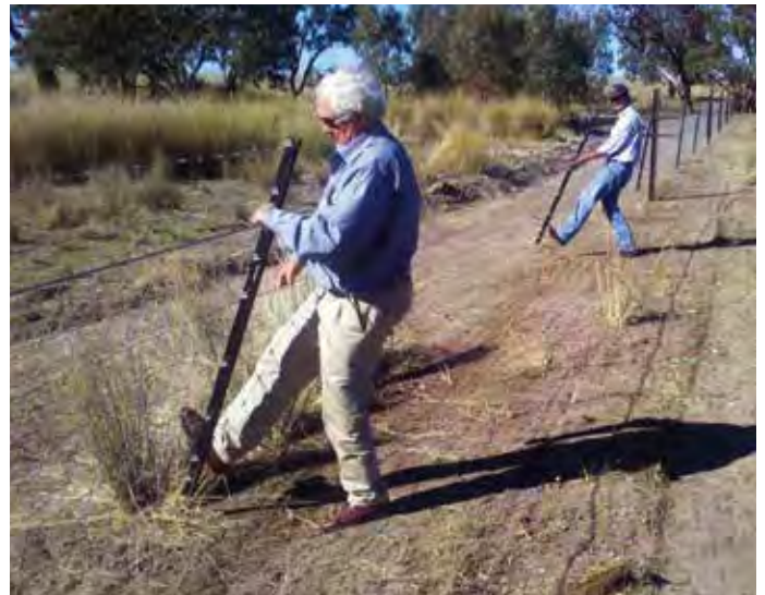
Fence in a floodway , suspended from a steel cable attached to heavy duty posts dug deep into the ground. Each fence is designed to lift up or fold over in the event of a flood.
