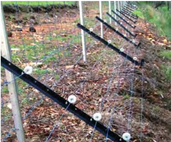
Sloping electric offset , being used in conjunction with an existing prefabricated wire fence.
