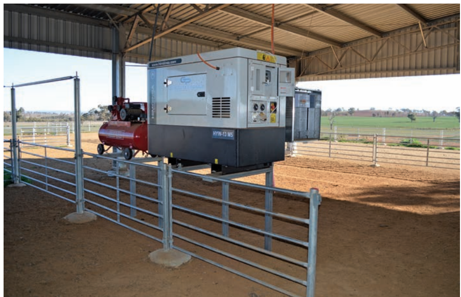
Diesel generator and air compressor.
