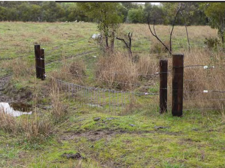
A chain-type floodgate forming part of the fenced section of the creek.
