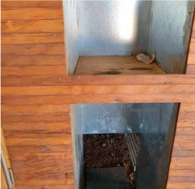
Figure 10: let go chute and shearer storage. The storage has a raised edge on the board side to stop falling objects and has a timber surface to reduce vibrations and wear on the shearer's tools (rubber could also be used).
