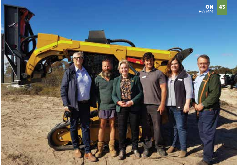
The AWI-funded Caterpillar skid steer loader with a hydraulic rock hammer used for installing fence strainers. Pictured are AWI director David Webster , SBF manager Craig Robins (obscured, driving the bobcat), SBF maintenance Paul Clune , WA Agriculture and Food Minister Alannah MacTiernan , WA Wild Dog Action Plan project manager Matthew Stadler , DIRPD Invasive Species director Victoria Aitken and AWI Vertebrate Pests program manager Ian Evans .
