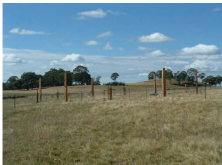
Above—A circular 'wagon wheel' water point under construction. The high posts allow hot wires to pass over the top of ten gateways that will open on to a central trough.
