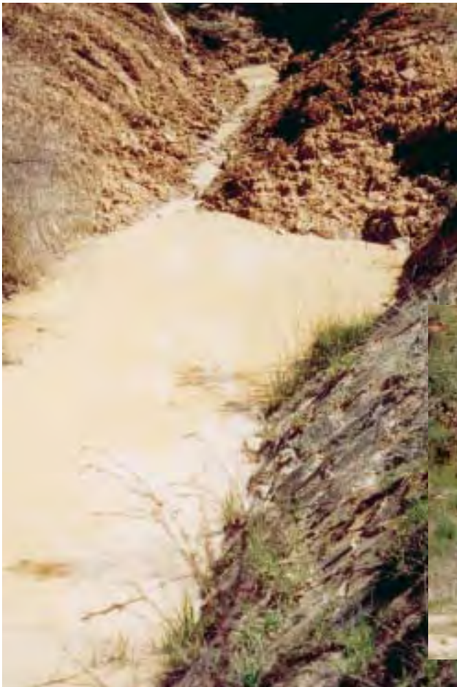
Left: A track has been built across this small stream with no attempt to stabilise the banks. As a result, the water is highly turbid and in the event of a flood, will erode the loose soil banks. Over time, this channel is likely to deepen as the sides and bed are scoured away. Photos Phil Price.
