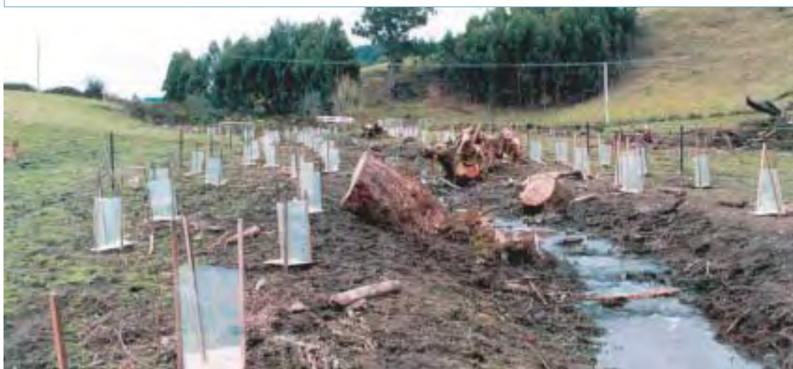
Although this small stream looks ‘messy’, it is on the road to recovery. It has recently had willows removed, stock access controlled and native species replanted as part of a restoration strategy. Photo Michael Askey-Doran.
