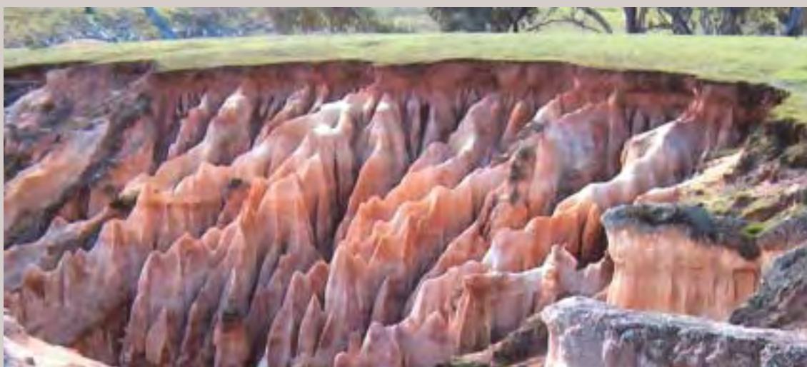
One of the side gullies on Bogolara. A combination of revegetation and 'hard' engineering will be used to address this erosion problem. Photo Gary Caitcheon.
