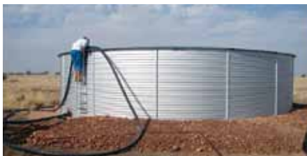
Figure 7 Storage tanks on Hillview
