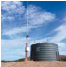
Figure 2 Water monitoring telemetry system set up on a tank.
