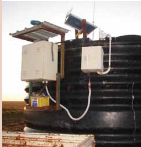
Figure 1 Telemetry infrastructure at water storage
