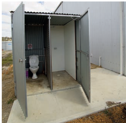
Ablution: A shower and toilet with a wash basin on the side wall is positioned to the side of the shed hardstand.
