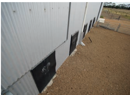
The wind tended to blow dust into the shed through the count-out doors, so rubber flaps were fitted over the openings. These are chained up for shearing.
