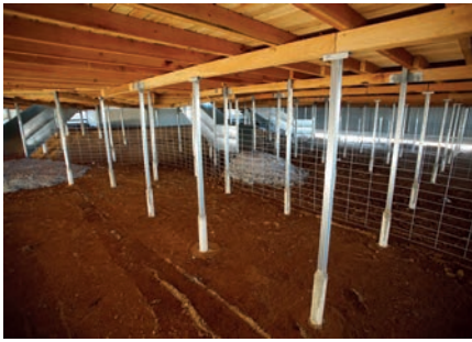
Corrosion protection: the bottom of support stumps are sleeved in PVC filled with brickies mortar to minimise the risk of corrosion.
